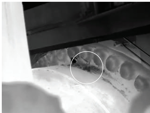
HBF leakage through GV #1
