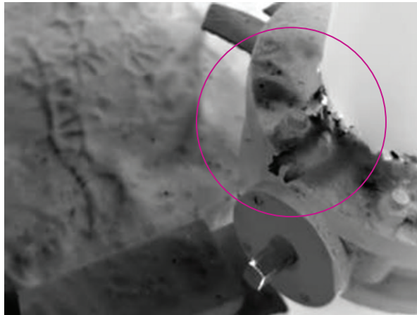
HSM pipe leakage at FCE #1
