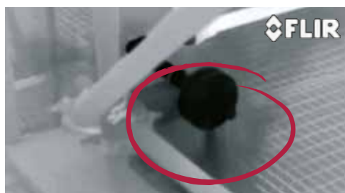
Gas leak is clearly visible on the thermal image.
